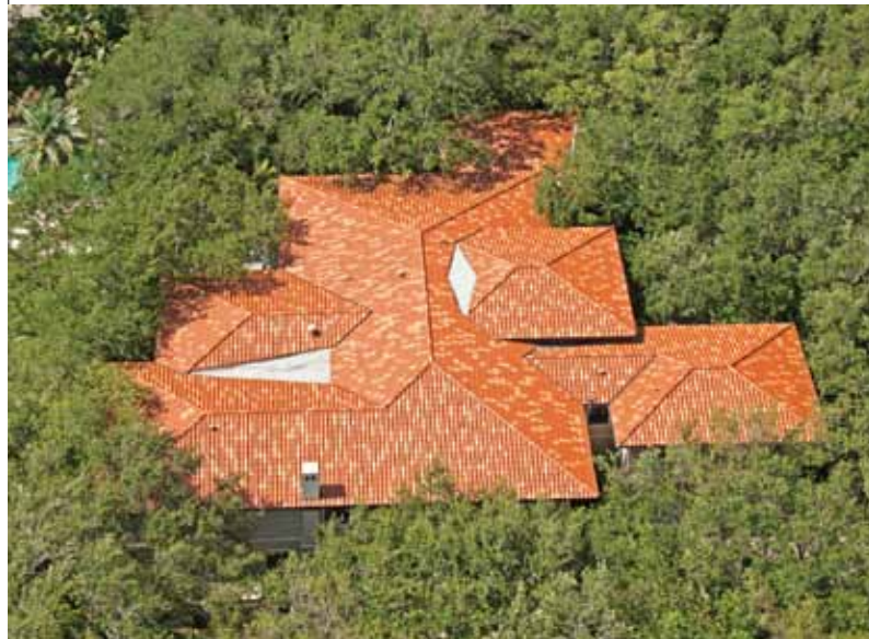
Located in Coral Gables, this home has a classic Spanish S clay tile roof with a custom blend of tile colors that gives it an authentic and individual style. The roof is complete with European half-round copper gutters.
