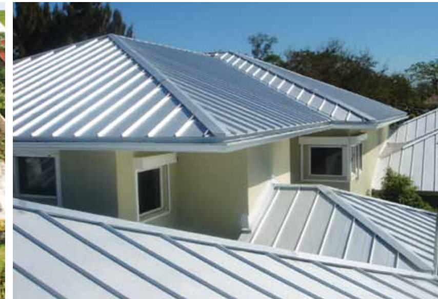
This Pinecrest home has a mechanically locked 1.5 standing seam metal roof with a mill finish. It is made from recyclable materials and has high reflectivity and thermal emission, making this roof energy efficient.
